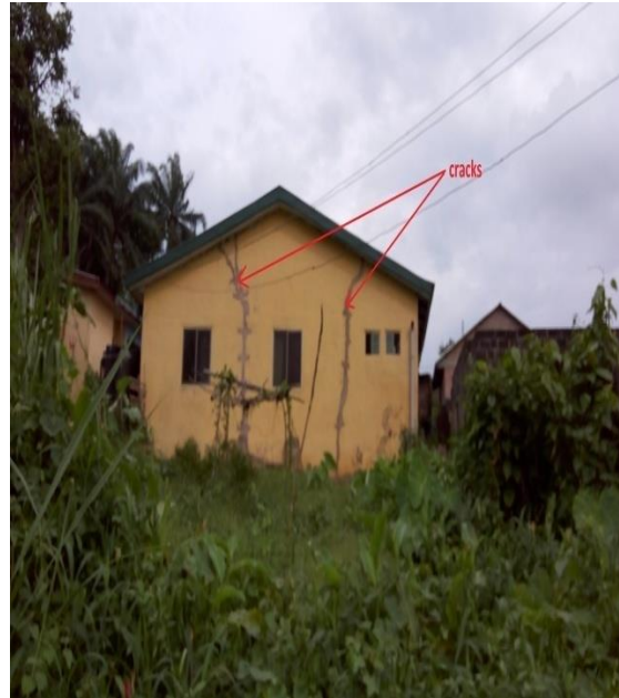
Fig.2: Cracks on walls of buildings
